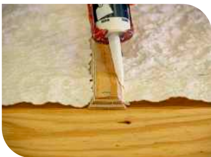
Sealing formliner with caulking – Uneven Edge
